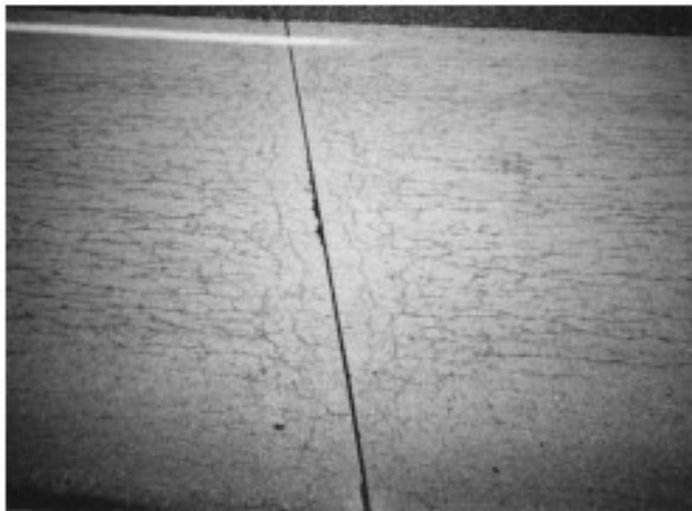
Fig. 4—Photograph of pavement affected by ASR. Typical longitudinal cracking is parallel to the slab free edges, with additional transverse cracks in the areas near the transverse joints.
