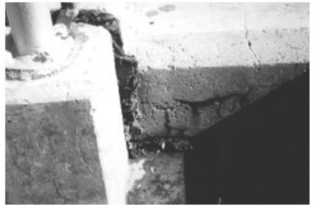
Fig. 5—Photograph showing closure of a joint and extrusion of joint-filling material due to ASR expansion.
